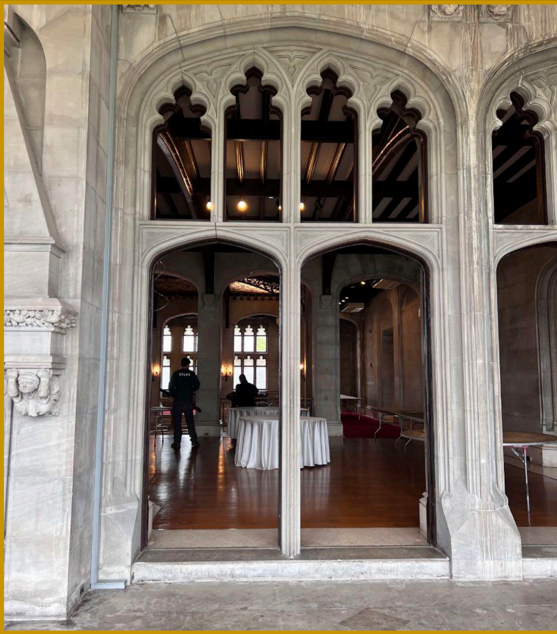
MISSING ARCHITECTURAL ELEMENTS AT LOCATION
