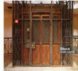
OLD ELEVATOR CAB DOOR W/ WINDOW REF
